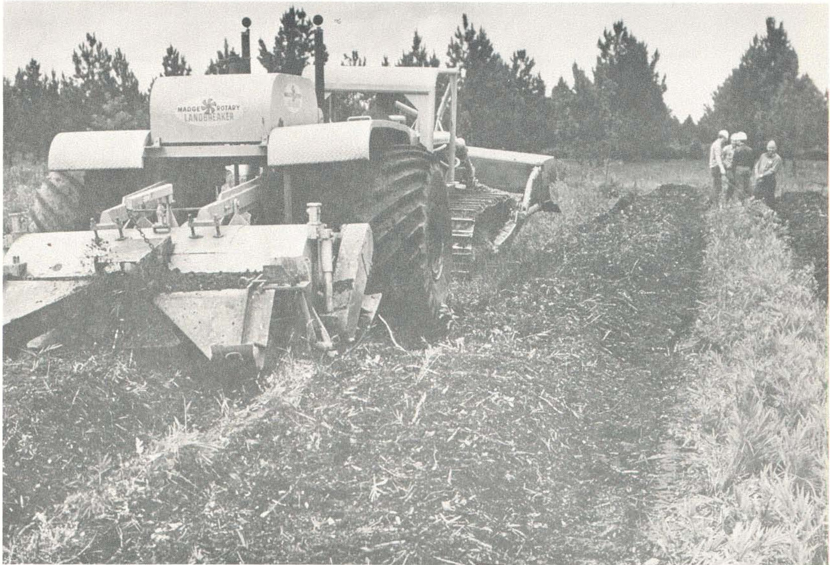
Intensive site preparation has become widely accepted. One of the most intensive operations is being done by Weyerhaeuser with this landbreaker. The beds are excellent for both pine and hardwood production.
